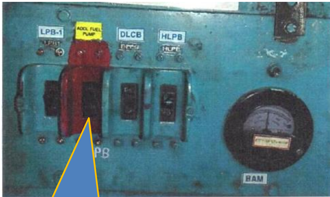
Additional Fuel Pump Breaker
