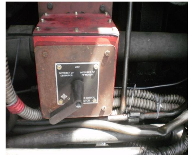
In Compressor Room
