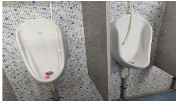
Cleaned urinals at Mysuru station
