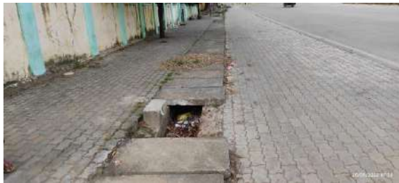
Shimoga colony drainage before
