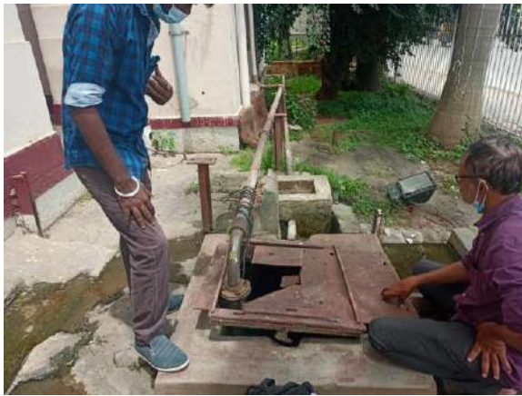
Inspection of water pump by HI at Mysuru
