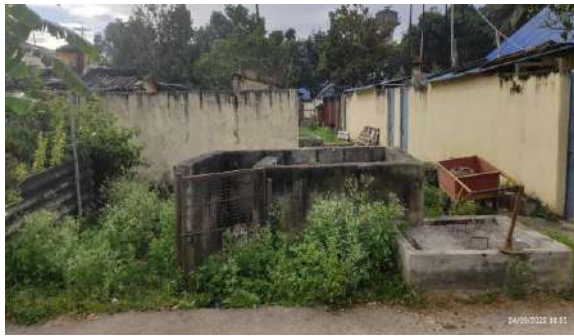
Garbage bin before cleaning at Shimoga colony
