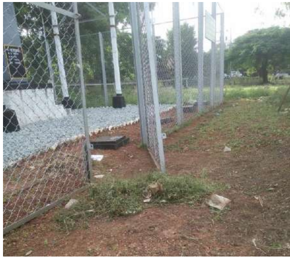
After cleaning outside Birur sub station
