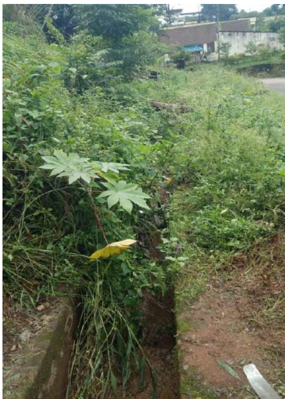
Sakaleshpur drainage before cleaning
