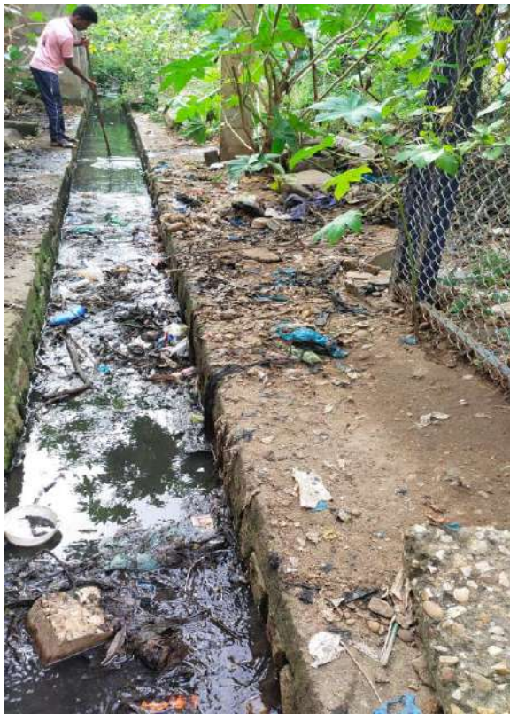
Sakaleshpur drainage before cleaning
