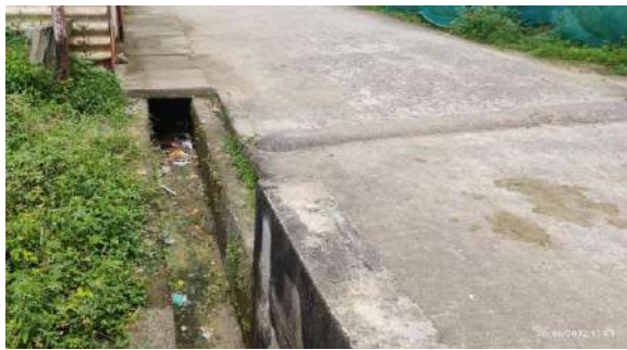
Before cleaning at Shimoga colony
