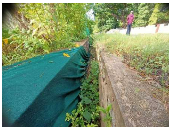
Mysuru colony open drain before cleaning
