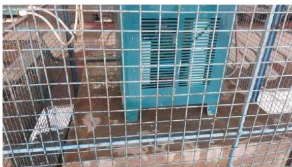
Water cooler -after cleaning at MYSURU station
