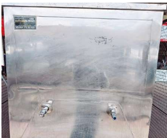
Water cooler after cleaning- ARASIKARE station
