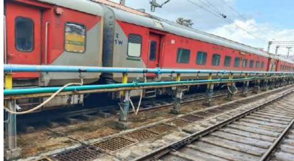
Proper positioning of hydrant pipes at Mysuru station
