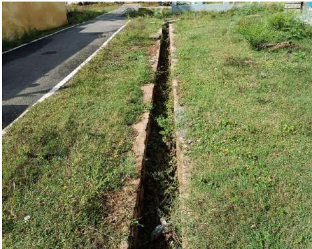
Arasikere colony drain before cleaning
