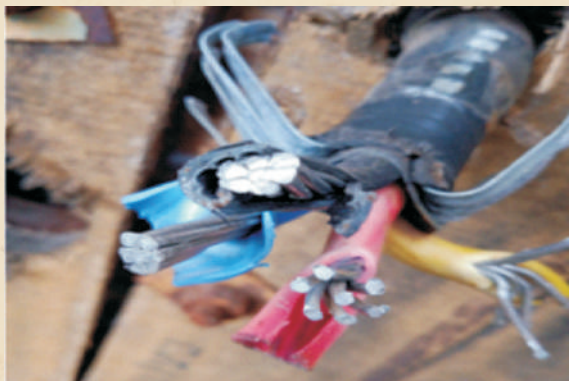
At Ends : 4 x 95 sqmm - 07 strands in each core.
